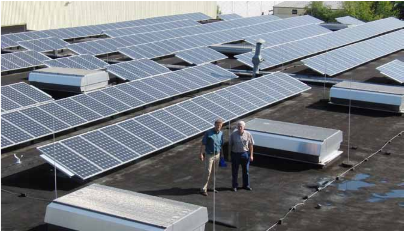
Solar panels at Elopak Speyer
