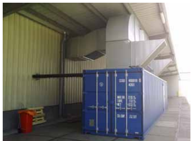
Elopak Terneuzen is also investigating the possibilities to replace the central heating system. Today's systems typically have an efficiency of about 90%, whereas the old system has an efficiency of only 60%. These figures show that a yearly CO 2 -reduction of 336 tons is well possible.
